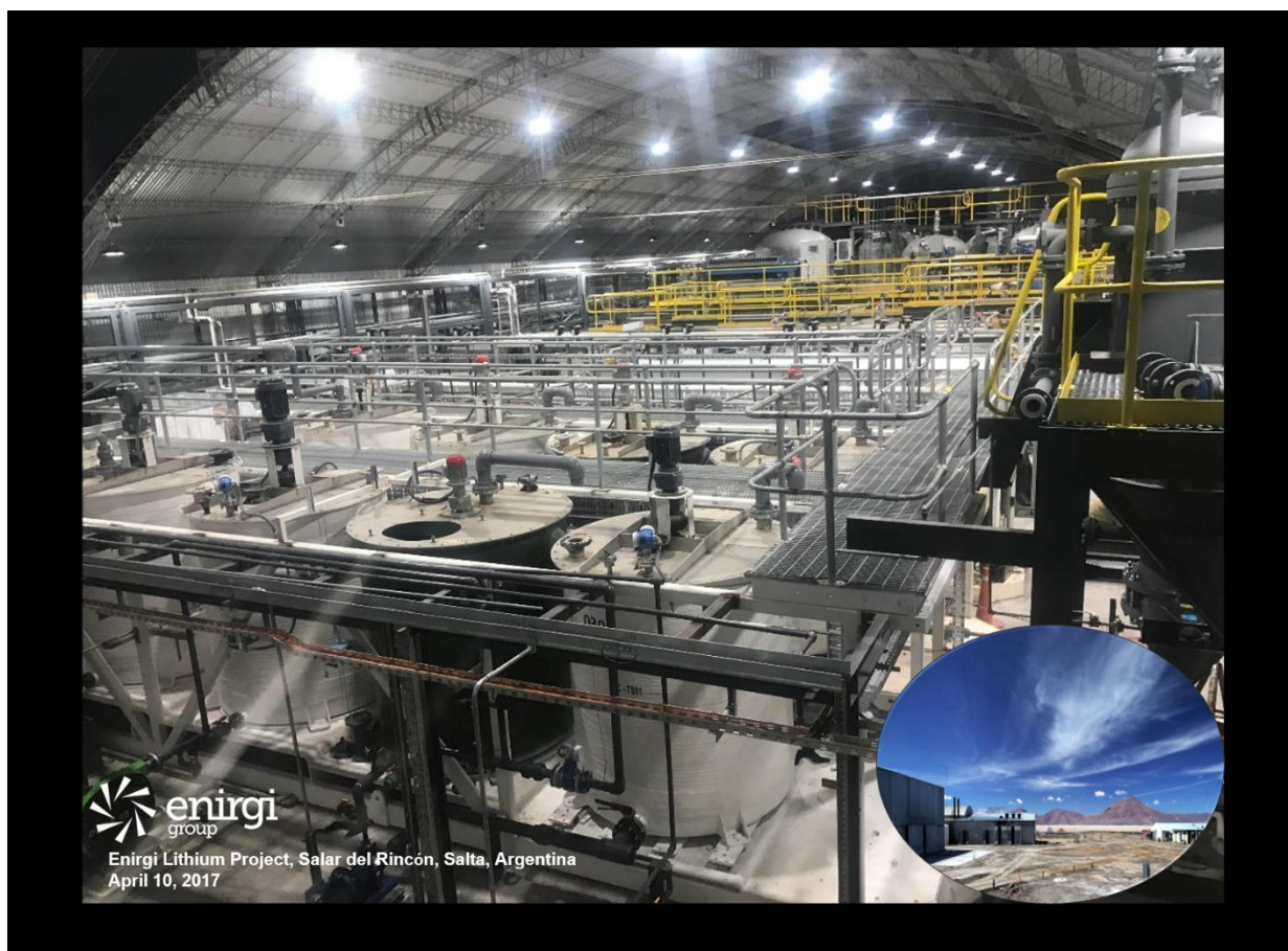
Figure 1: View from the Control Room, Southern Building, DXP Plant, Enirgi Lithium Project
